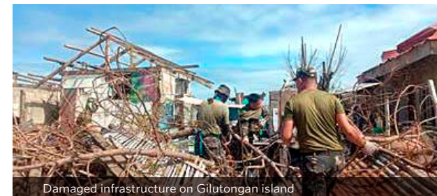
Damaged infrastructure on Gilutongan island
